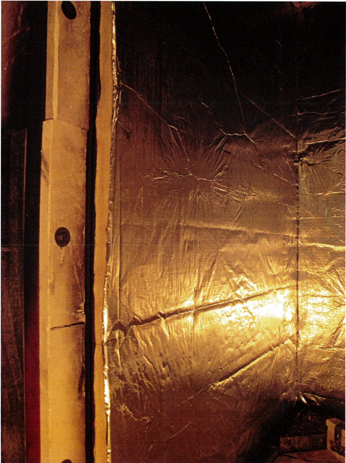
Photo no 2 Prior to test “CR-DUCT”
